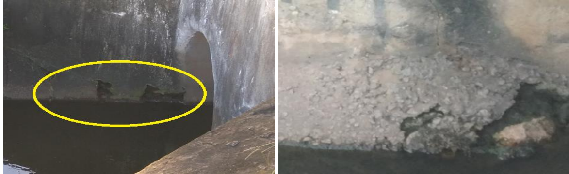
FIGURE 04: Erosion and cavitation wear at points near the culverts.
