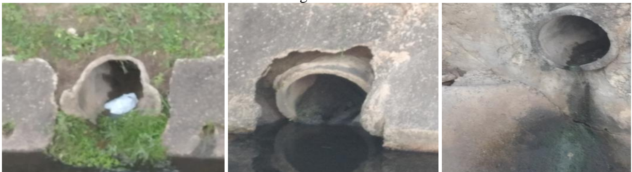
FIGURE 05: Erosion and cavitation wear at the connection between the rainwater galleries and the urban drainage channel.
