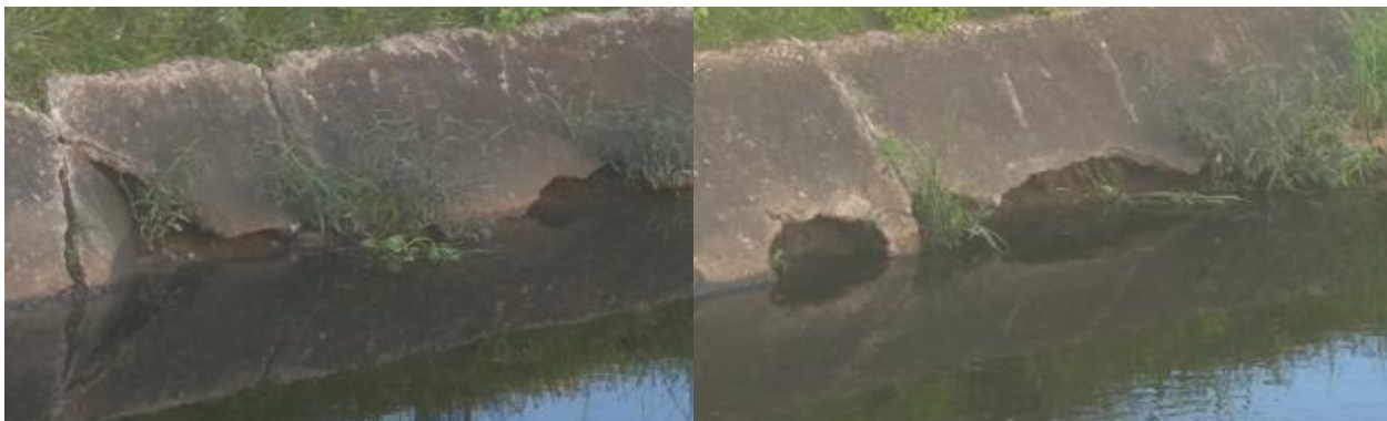
FIGURE 6: Erosion and cavitation wear on the side walls of the channel.
